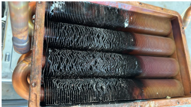
A copper heat exchanger with hard water damage caused by scale.
