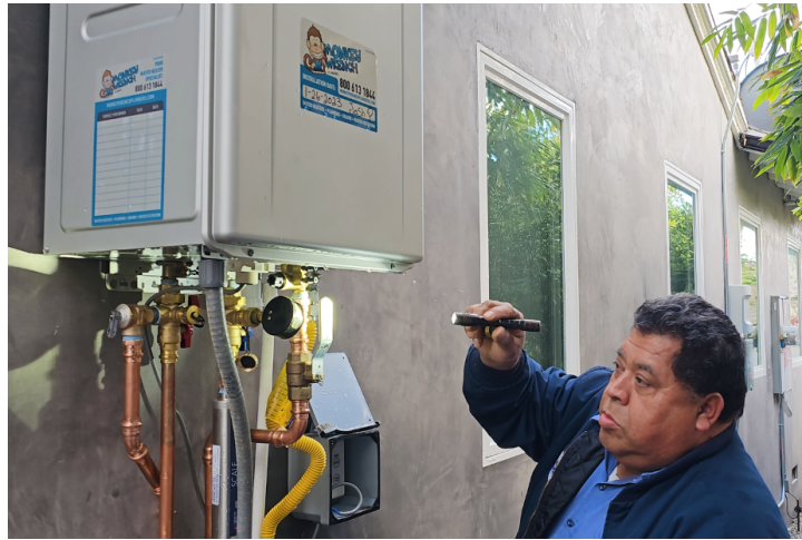
A Monkey Wrench technician inspects a Noritz tankless water heater with a flashlight.
