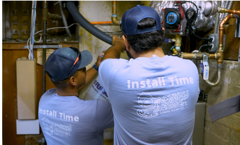
Two Monkey Wrench technicians in the process of installing a tankless water heater.
