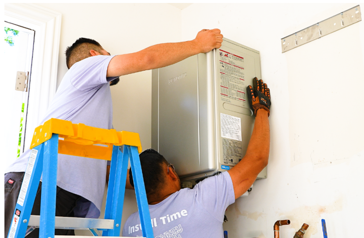
Two Monkey Wrench technicians preparing to mount a Noritz tankless water heater.
